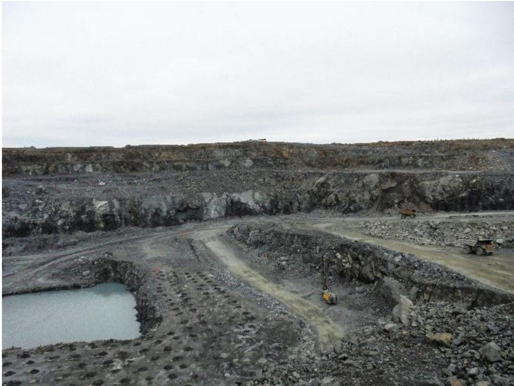
Fig. 17-1-10. selected area for following blasting in the open pit (photo: Ch. Bovier).
